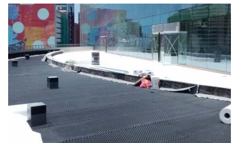
The installed materials are the Protection Mat SSM 45, the drainage element Floradrain® FD 40-E, Filter Sheet TG and Inspection Chambers KS 6.
